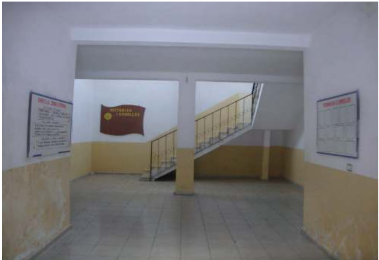
The entry hall – large but empty and in need of repair.
